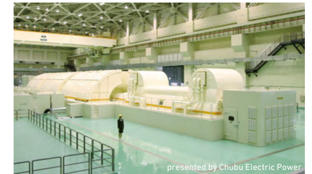
presented by Chubu Electric Power 1570MVA Nuclear Turbine Generator
