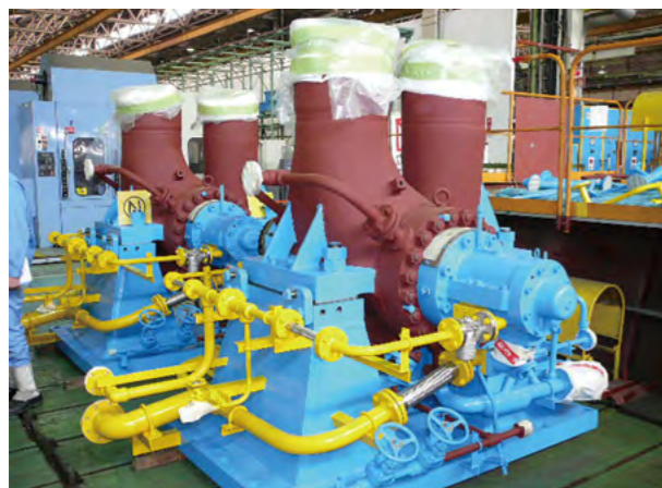
Main Feedwater Pump
