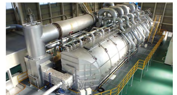
Combustion Test Facility (4t/h)
