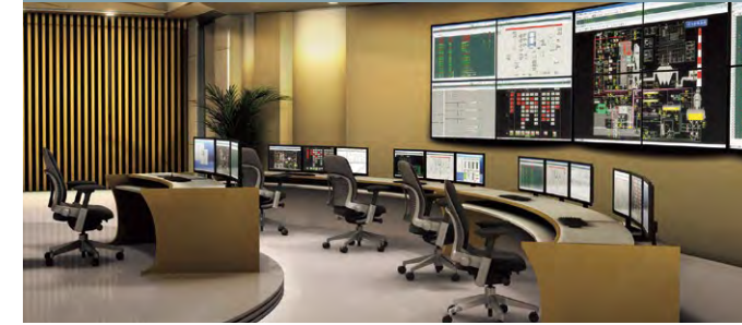
Plant Control System
